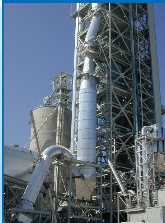
Gas Conditioning Tower
